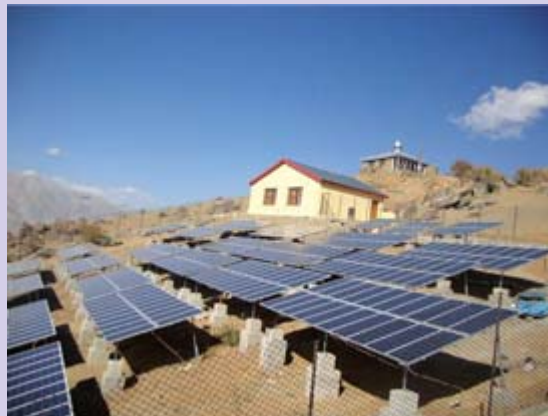
40 kWp SPV Power Plant at Yurbaltak Kargil, Jammu & Kashmir
