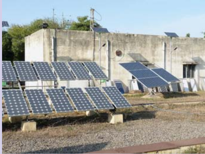
Solar PV Test Bed at Solar Energy Centre
