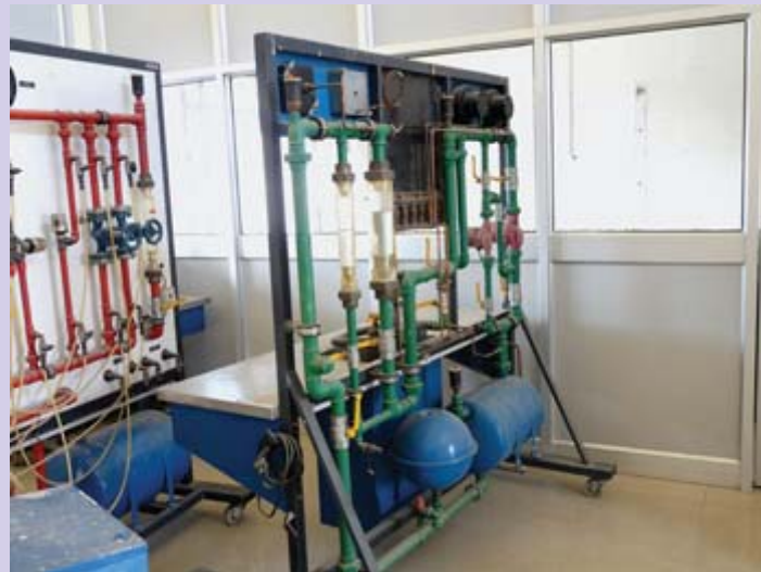
Solar Air Conditioning Laboratory at Solar Energy Centre
