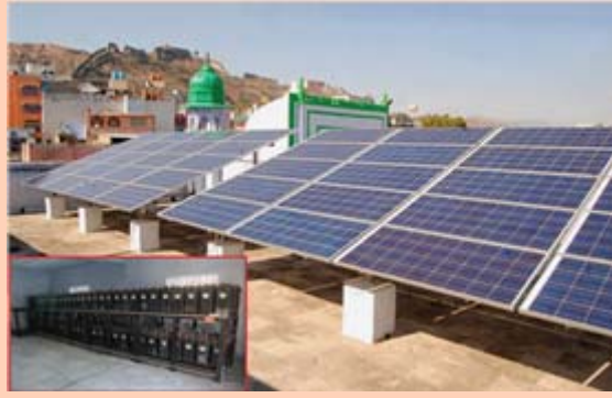
SPV Power Plant at Dargah Khawaja Garib Nawaj, Ajmer, Rajasthan, under Special Area Demonstration Project Programme
