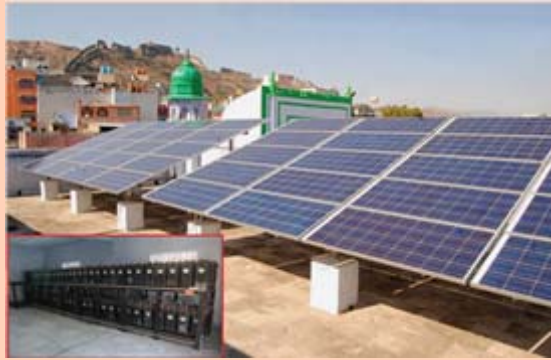
SPV Power Plant at Rajbhawan, Jaipur, Rajasthan, under Special Area Demonstration Project Programme
