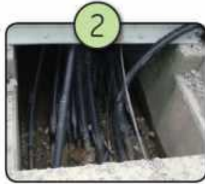
Traditional cable trenches
