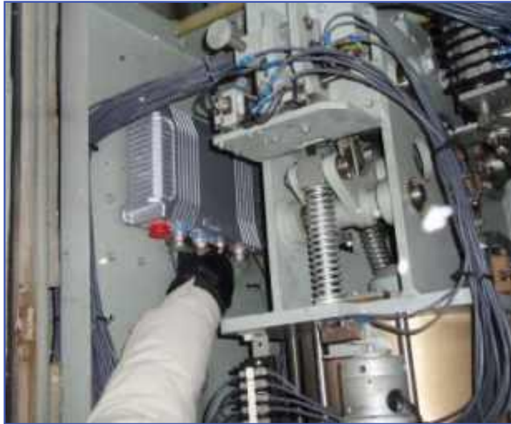
Internal, old oil-type Circuit Breaker
