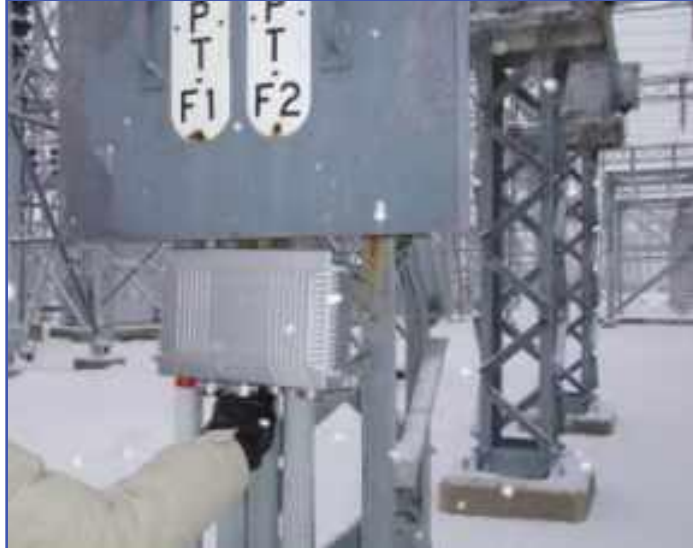
External, below VT marshalling box
