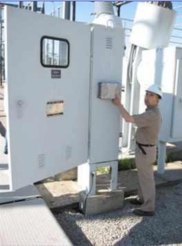
External, on a Circuit Breaker
