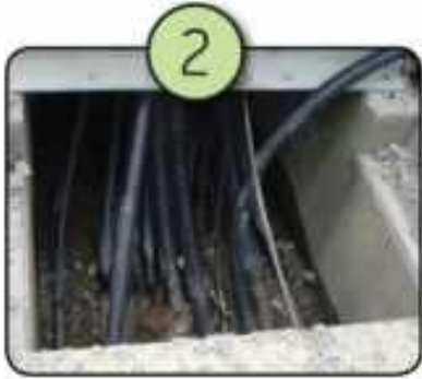
Traditional Cable Trench
