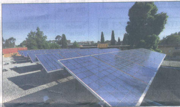
■ Solar panels are shown on top of a housing complex in California, United States
